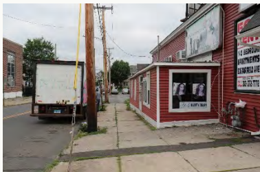
Delivery trucks service from street, conc, sidewalk in poor condition, guy wires and utility poles in walk
